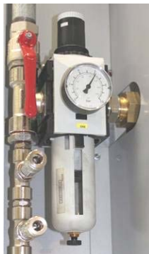
Compressed air supply
