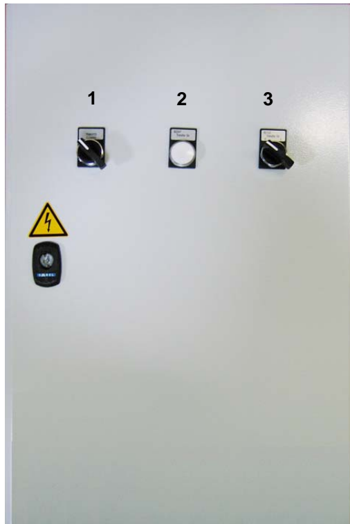
PT Control - front view
