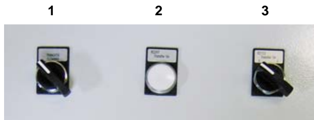
PT Control - switching on
